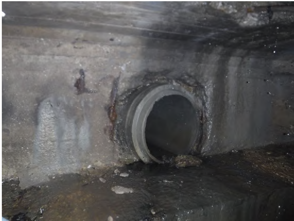
Figure 64 - STA. 20+18 18" Concrete and infiltration.
