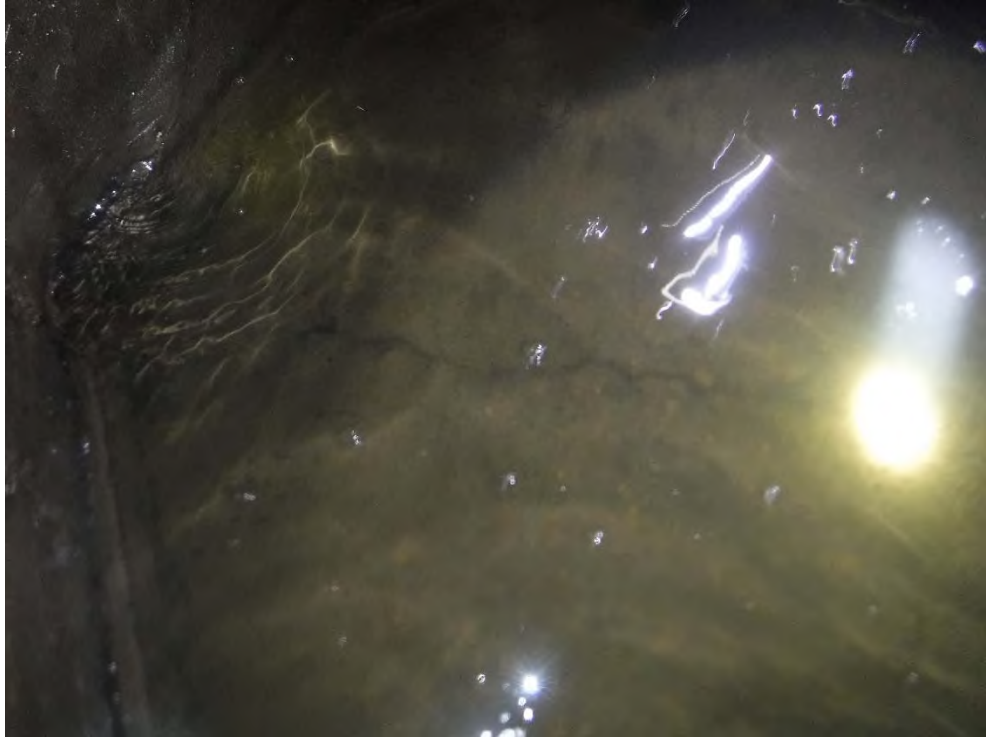
Figure 25 - STA. 16+02, diagonal floor crack.
