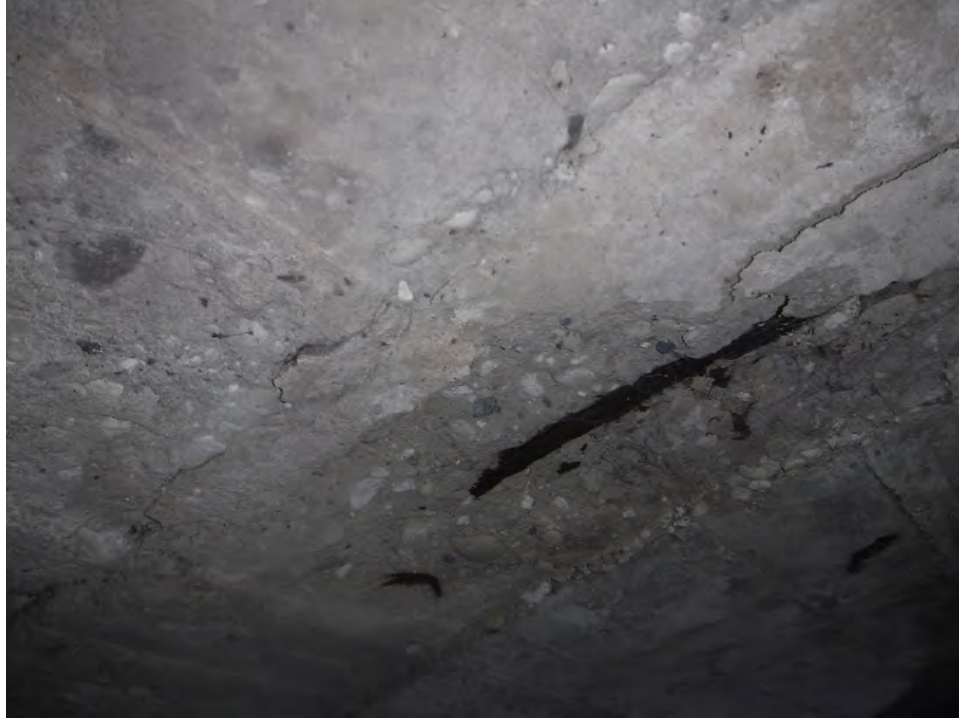
Figure 75 - STA. 21+00 construction joint failure at ceiling.
