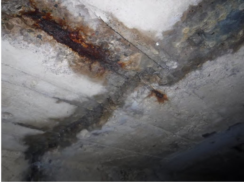
Figure 85 - STA. 22+30 ceiling failure.
