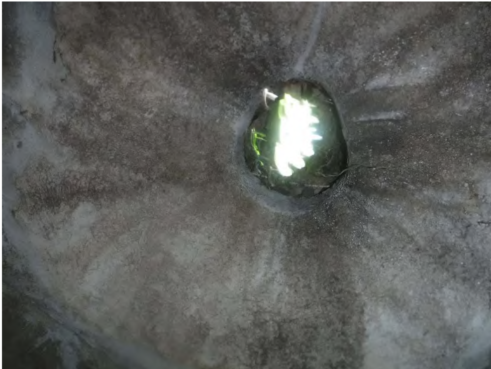
Figure 8 – STA. 10+55, storm inlet.
