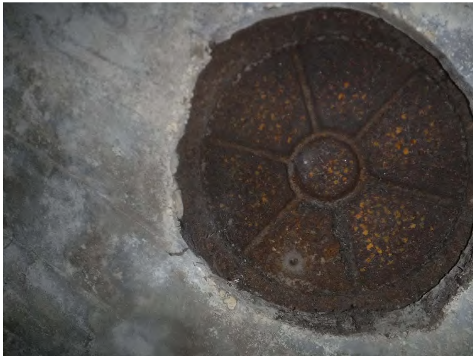
Figure 6 – STA. 10+25, Sealed Manhole.
