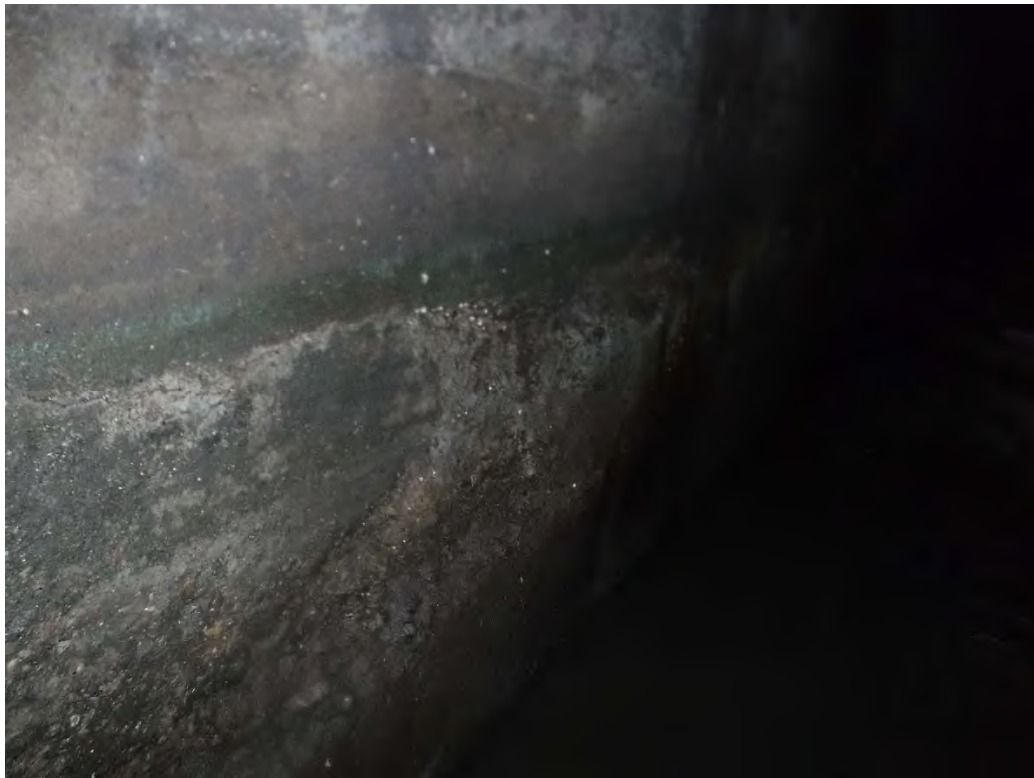
Figure 49 - STA. 18+65 Horizontal crack.
