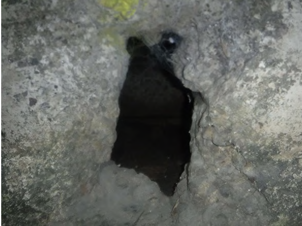
Figure 87 - STA. 22+83 break in inlet.
