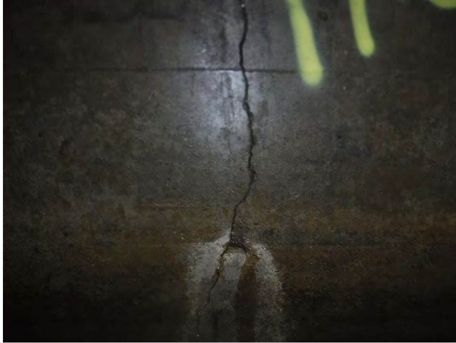
Figure 29 - STA. 17+05 wall crack.
