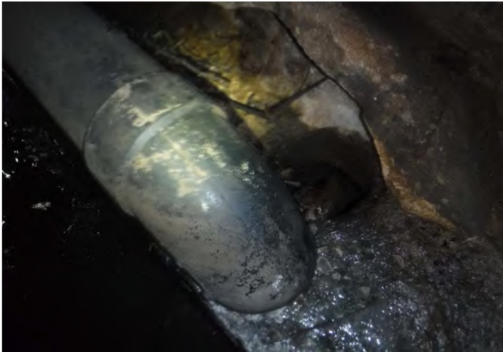
Figure 11 – Isolated failure: hole into sanitary sewer encasement.
