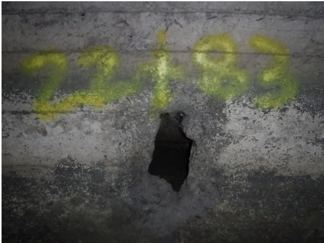
Figure 86 - STA. 22+83 break in inlet.
