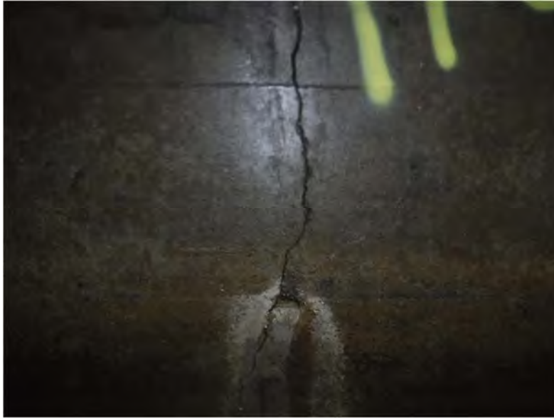
Figure 13 - STA. 17+05 wall crack.
