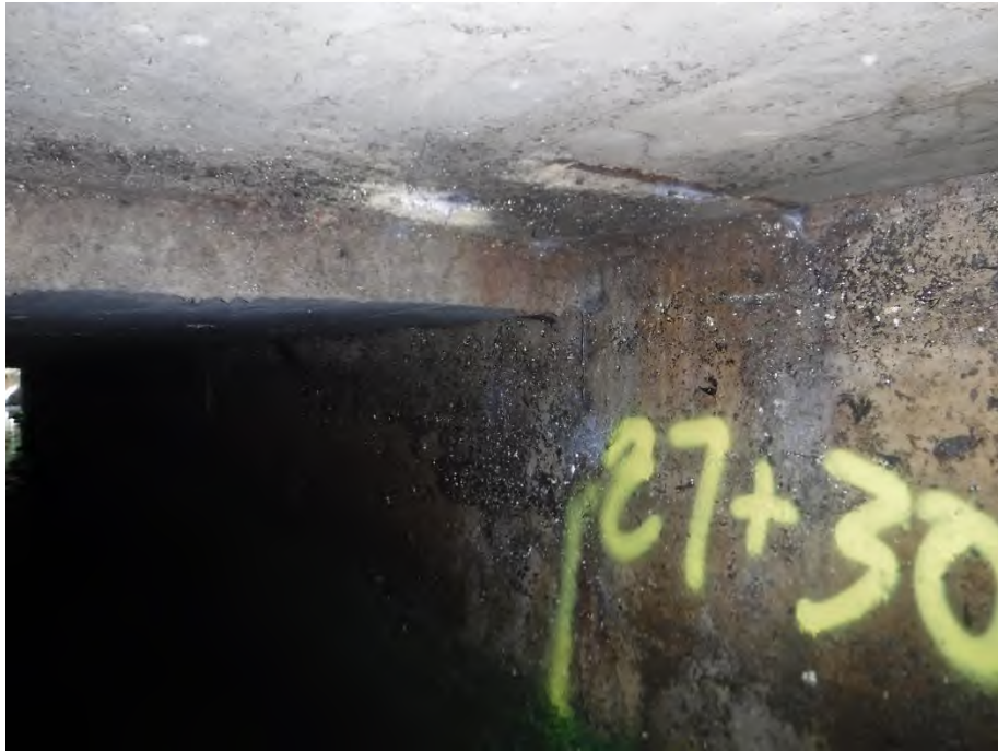
Figure 94 - STA. 27+30 new ceiling and adjacent delamination.
