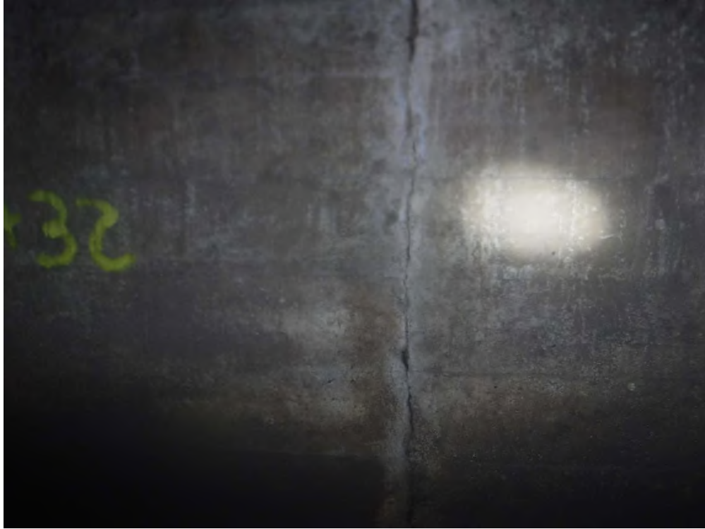
Figure 7 – STA. 10+30. Construction joint recommended grout repair.
