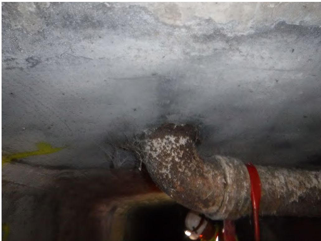
Figure 82 - STA. 21+32 ceiling delamination.
