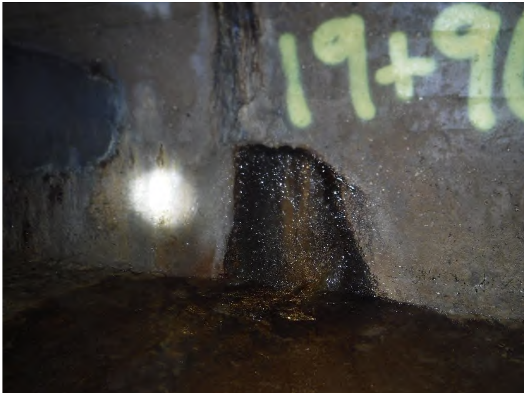
Figure 60 - STA. 19+96 construction joint with 3/4" opening.
