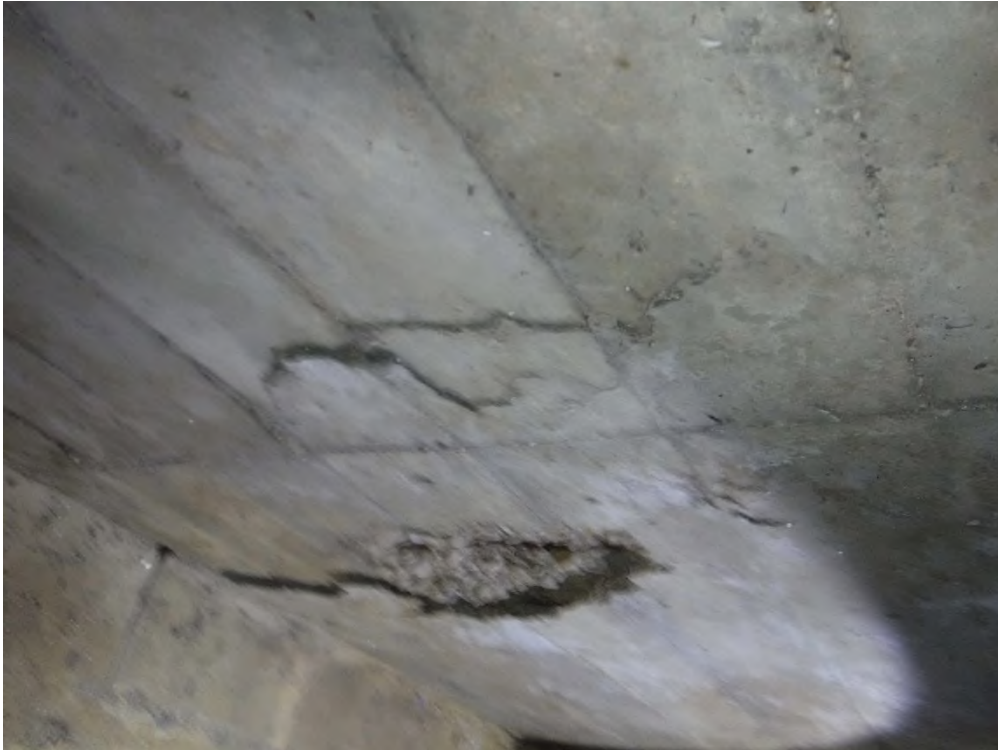
Figure 92 - STA. 24+36 ceiling failure.
