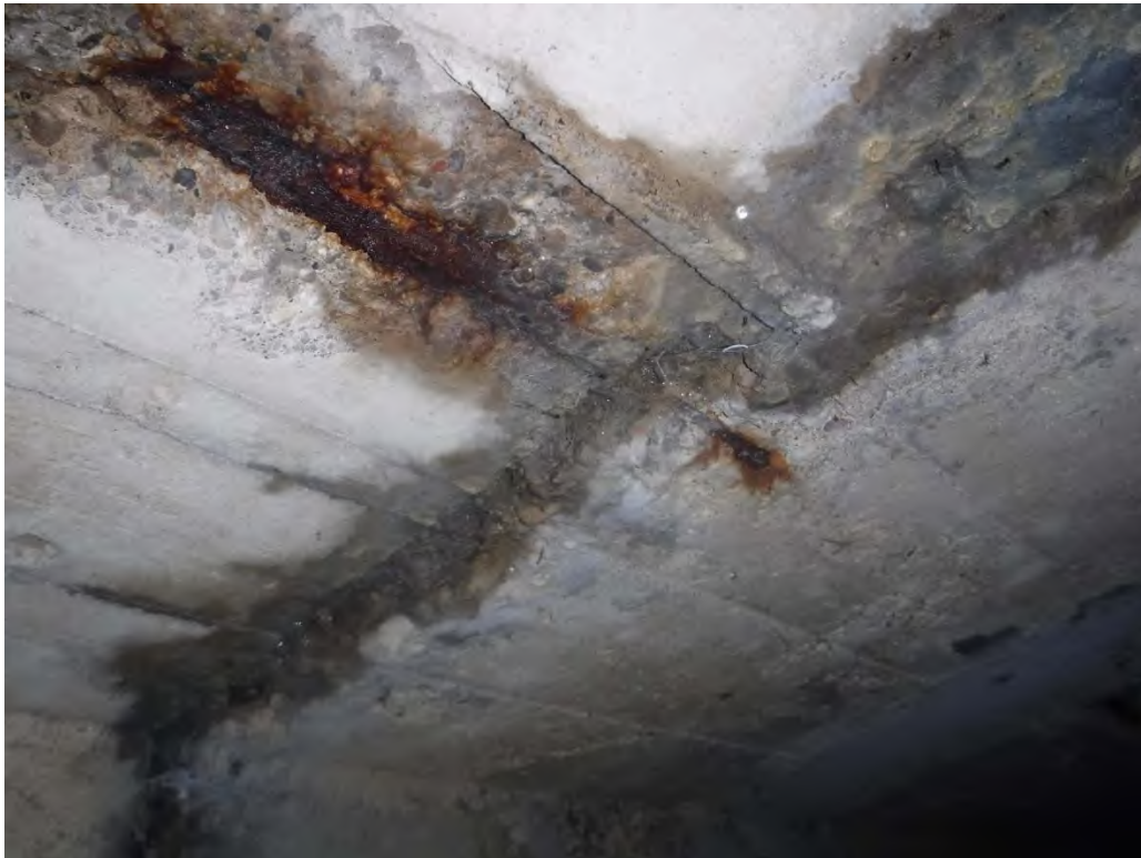
Figure 14 - STA. 22+30 ceiling failure with exposed rebar.
