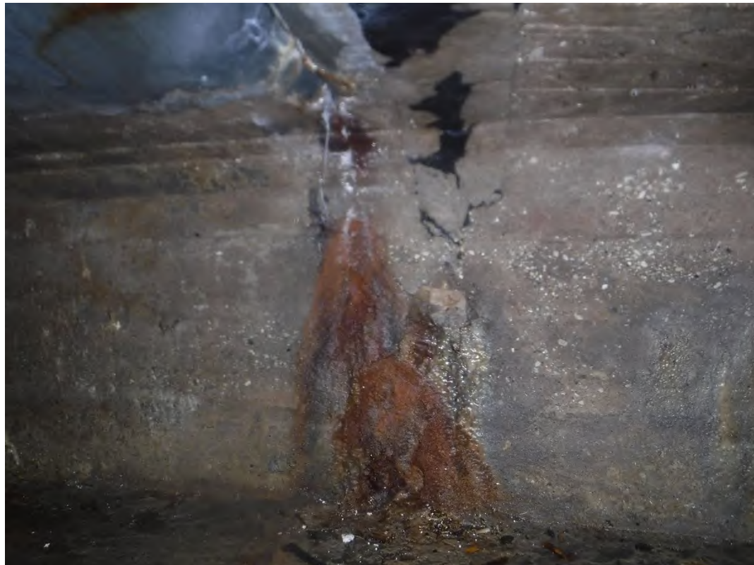
Figure 62 - STA. 20+00 ceiling delamination and infiltration.
