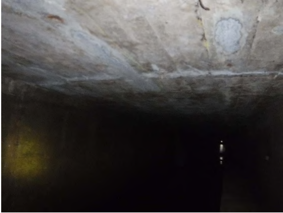
Figure 13 - STA. 11+28, ceiling delamination.
