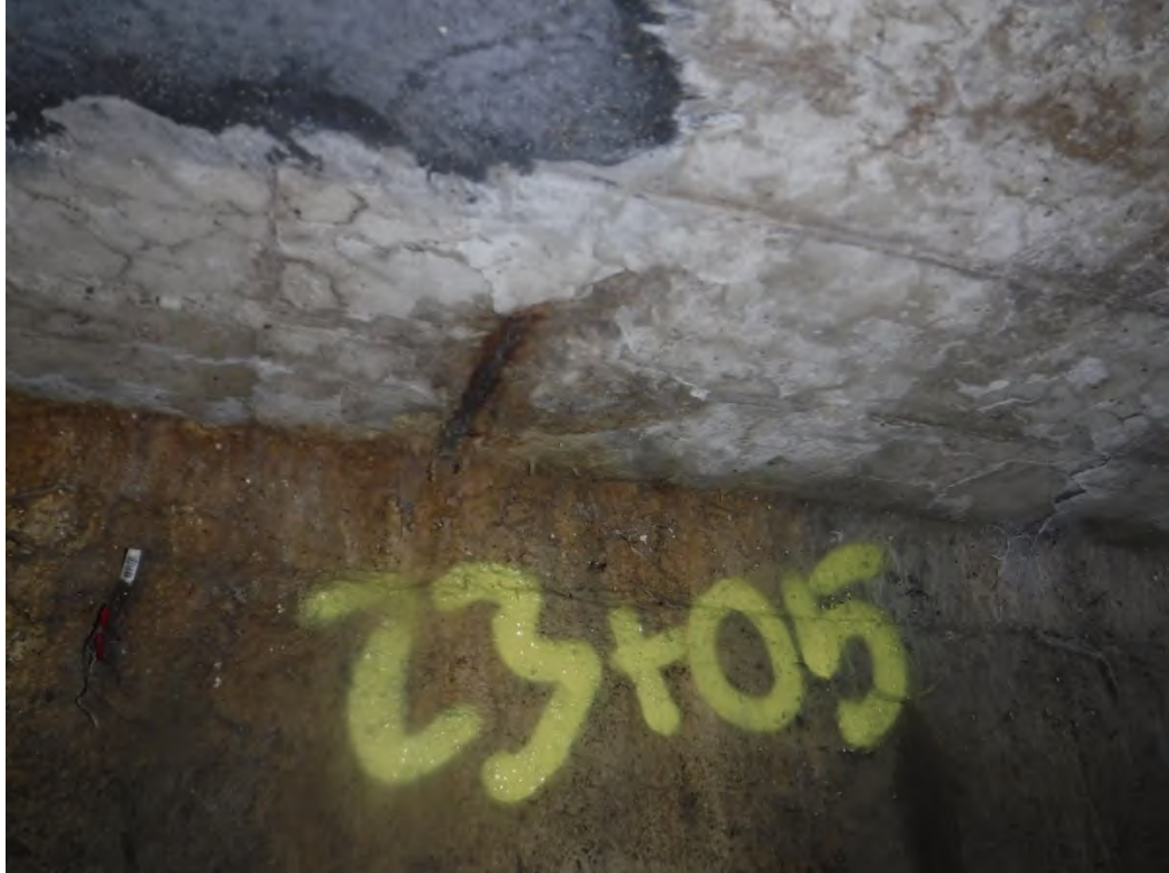
Figure 89 - STA. 23+05 ceiling delamination.
