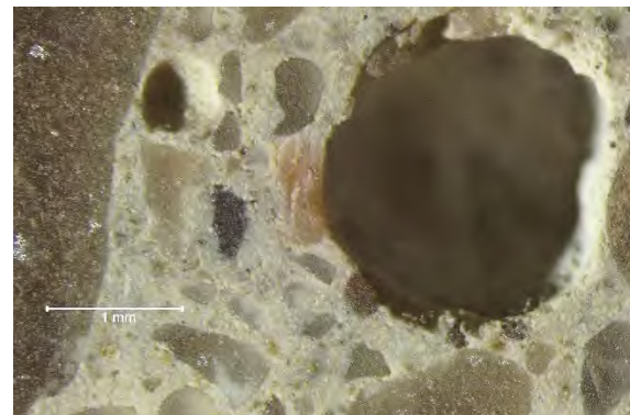
Magnification: 32x Description: Hardened air void system
