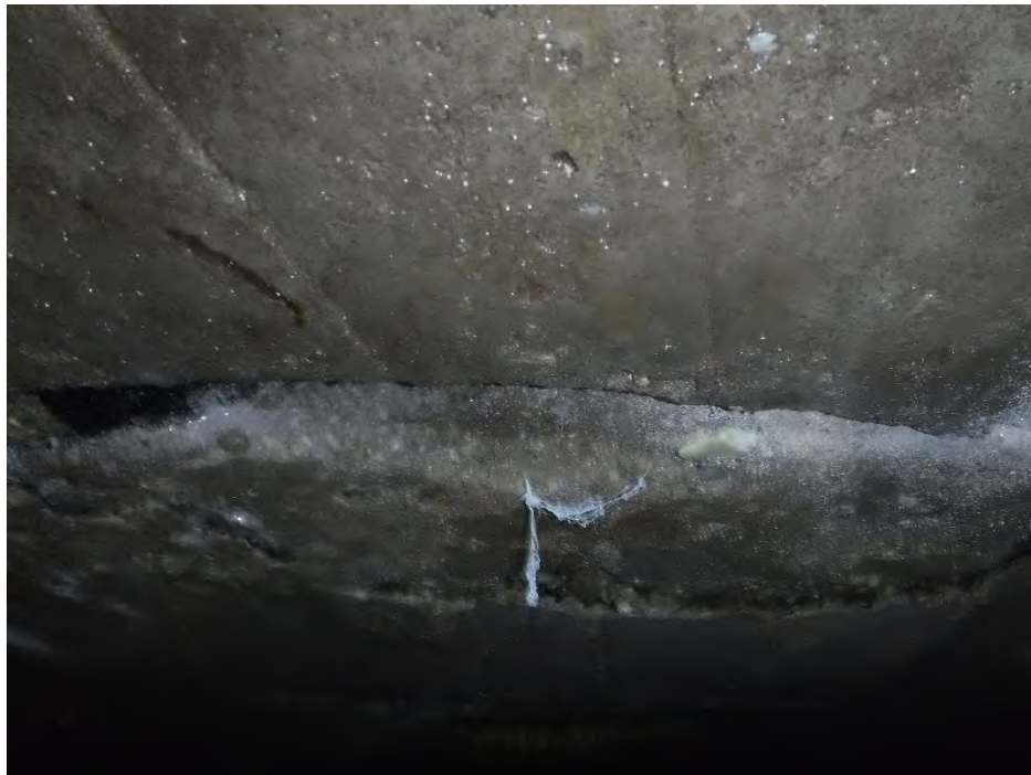
Figure 68 - STA. 20+45 to 20+59 ceiling failure.
