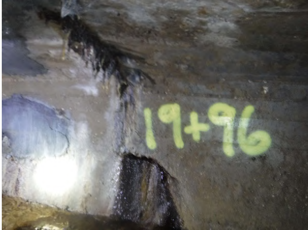
Figure 61- STA. 19+96 construction joint with 3/4" opening.
