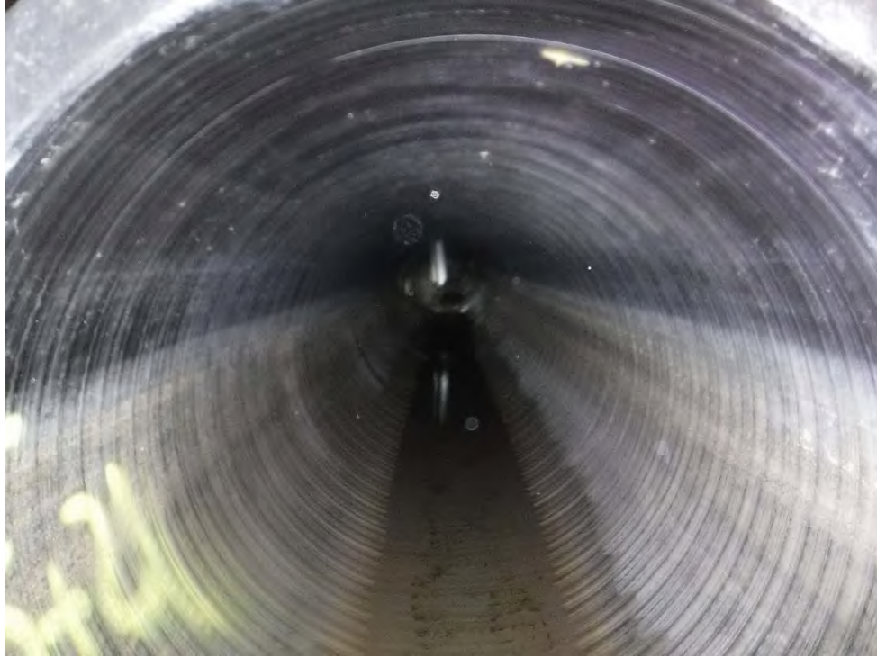
Figure 15 - 48" storm sewer lining in failure.
