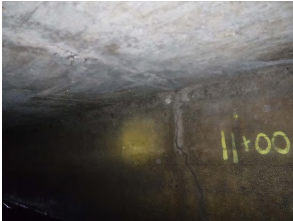
Figure 12 - STA. 11+00, recommend grout repair.
