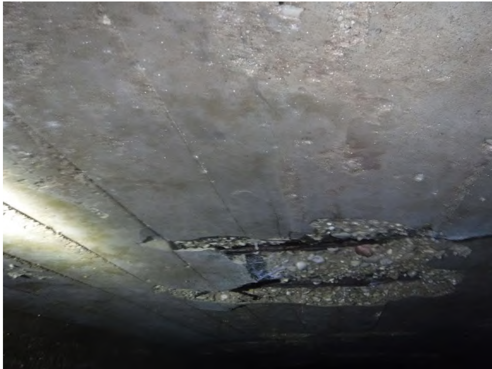
Figure 66 - STA. 20+45 ceiling failure.
