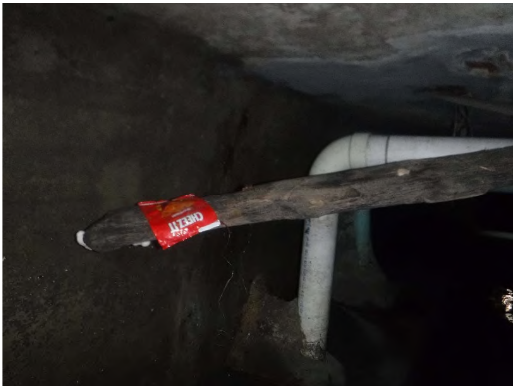
Figure 37 - STA. 17+92 connection and debris.
