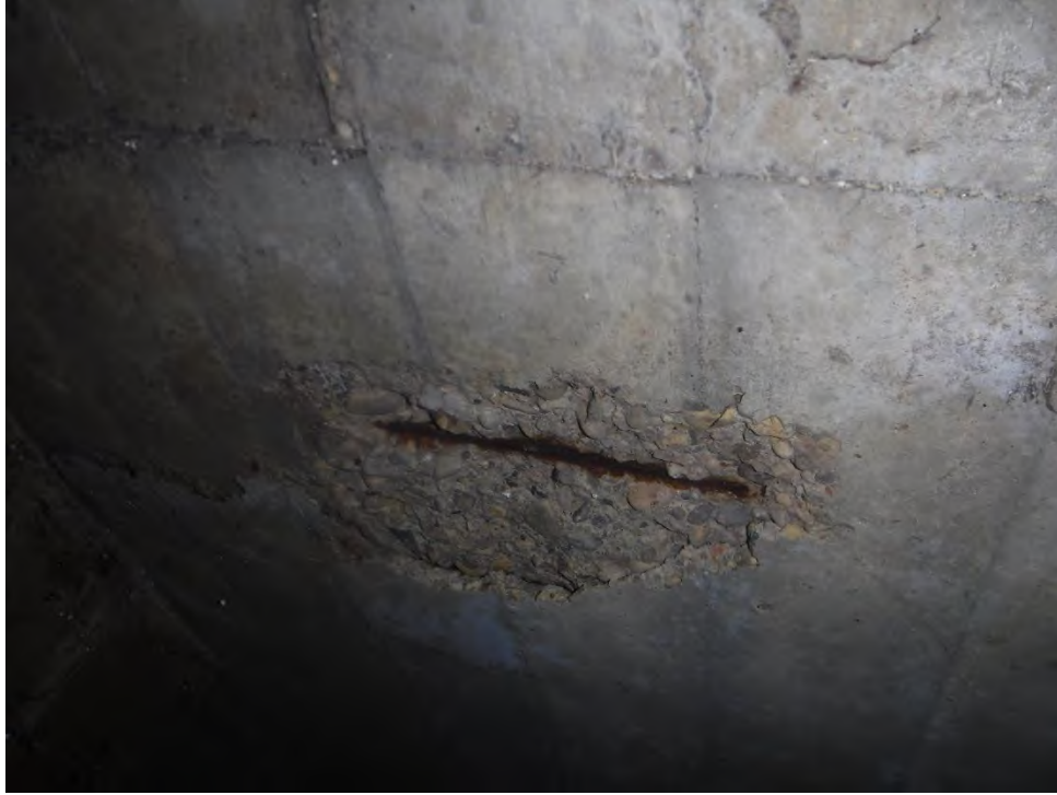
Figure 93 - STA. 24+36 ceiling failure.
