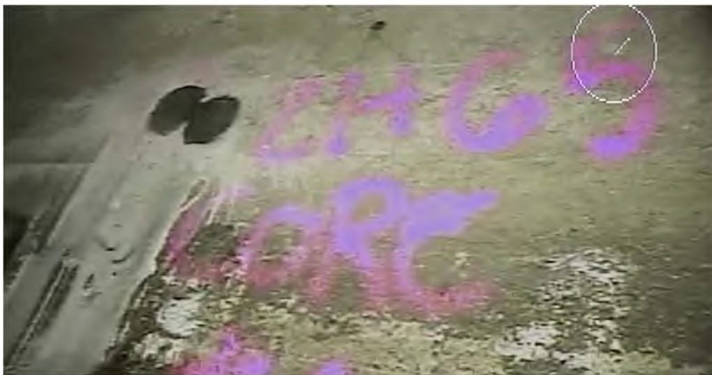
Figure 8 – Core samples patched at Station 21+65. Image is from the televising video.
