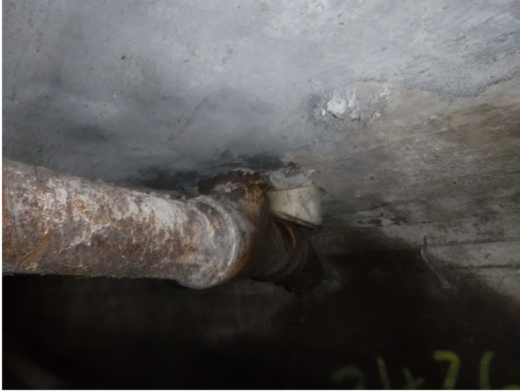
Figure 81 - STA. 21+32 ceiling delamination.
