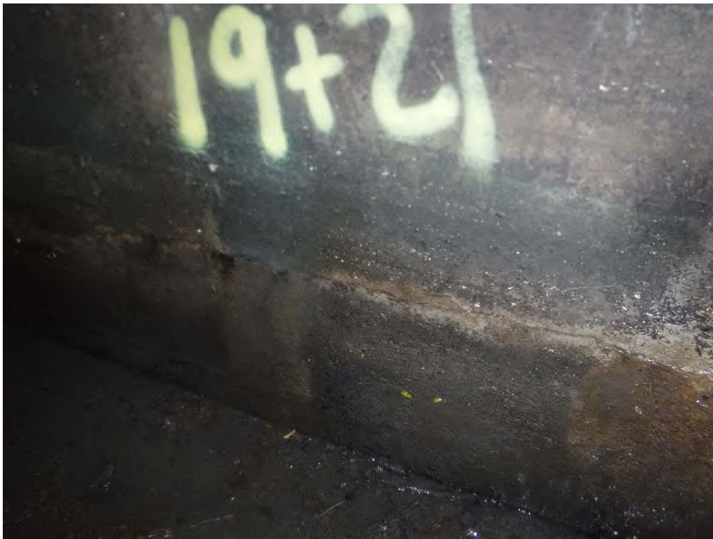
Figure 53 - STA. 19+35 horizontal crack.
