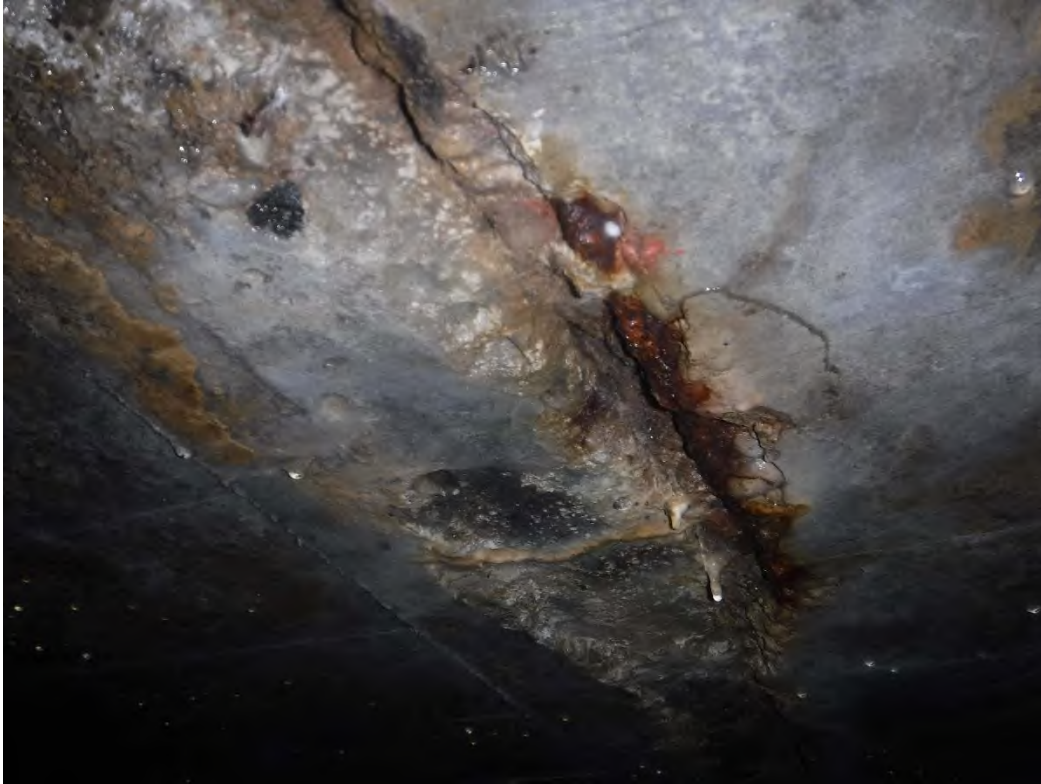
Figure 36 - STA. 17+60 grout repair needed.
