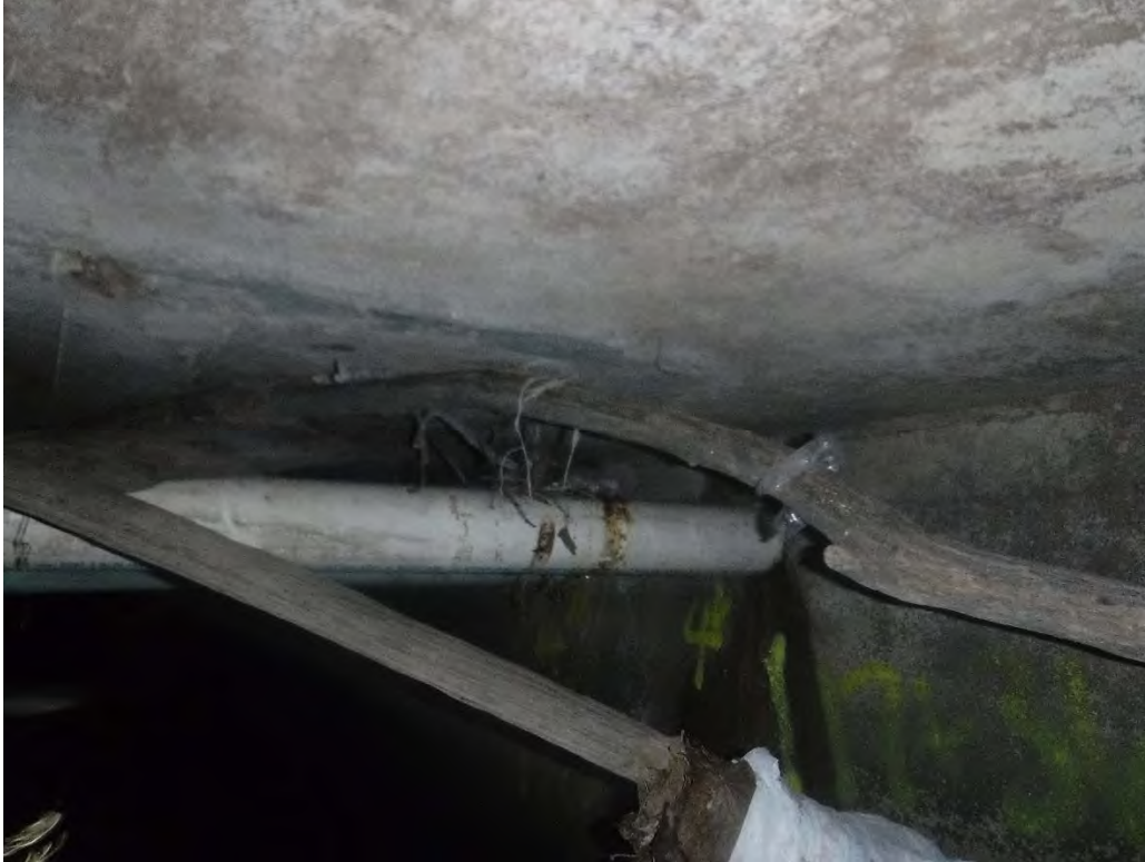
Figure 38 - STA. 17+92 connection and debris.
