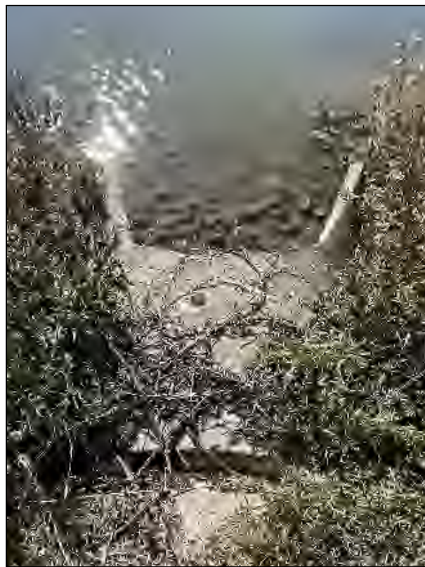
1. REPAIR EXISTING ENDWALL ON ROCKLAND POND OUTFALL FOLLOWING JOINT TIES DETAIL ON SHEET C507
